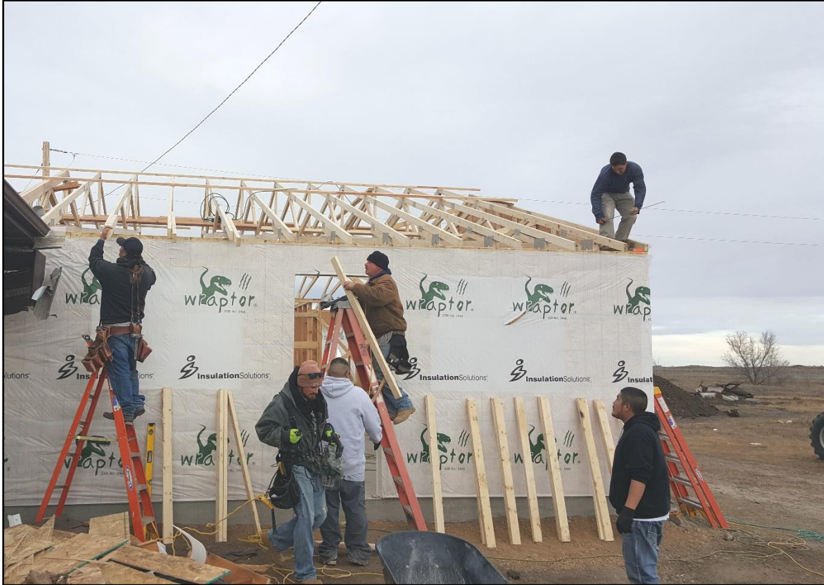
Nishu C Store expanding. The construction on this part of the store is complete, but work is still being done on the inside. Grand Opening date is unknown at this time. More in the News Journal next month.
