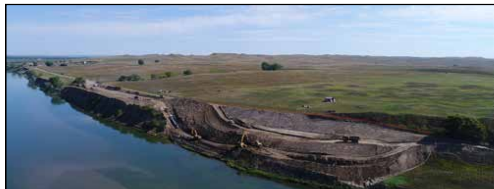
Aerial view of the bank stabilization project at Double Ditch on Aug 22 (Photo Dwayne Walker SHSND)
