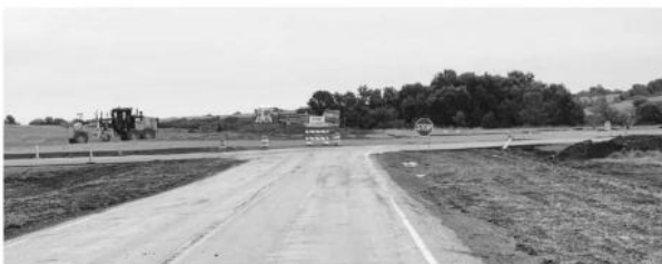
Construction of roundabout near Mandaree, at the junction of highway 22 and highway 73.
