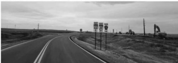
Construction of roundabout near New Town at the junction of highway 23 and highway 8.
